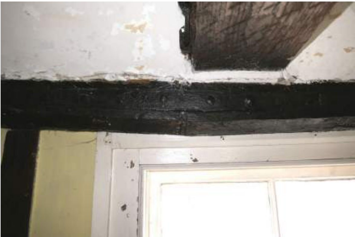
Photograph 45 Detail of plated scarf-joint in north-western wall-plate in bedroom 4. Photograph taken facing north-west.
