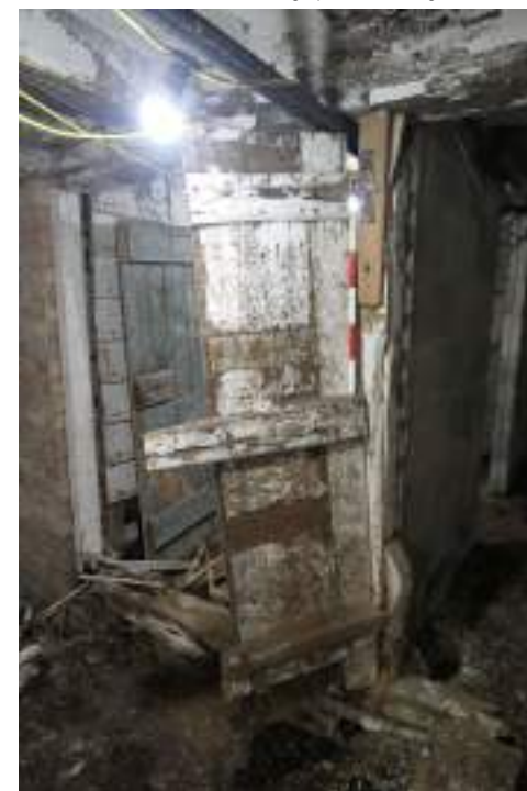
EEX62136_PhotoGraph_244 Detail of delapidated planked door in basement. Photograph taken facing north.
