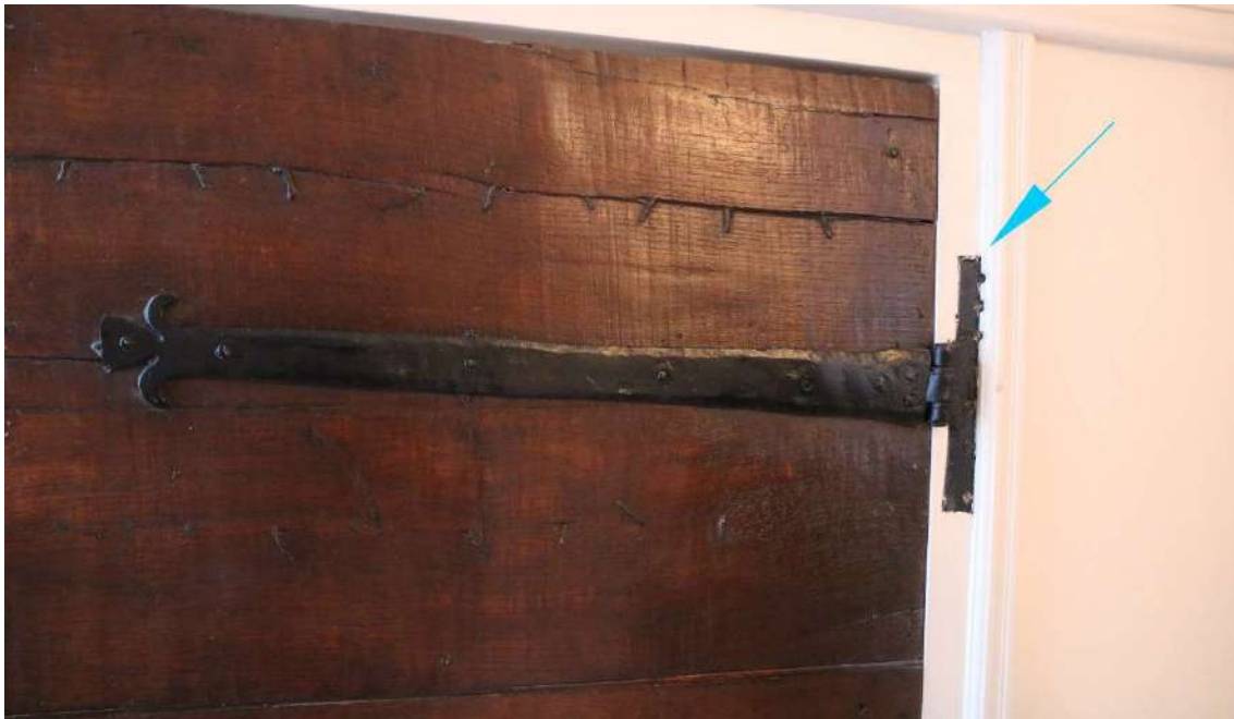
Photograph 35 Detail of strap hinge on door in south-eastern wall of bedroom 4. Blue arrow highlighting the architrave sealing the plate of the hinge Photograph taken facing south-east.
